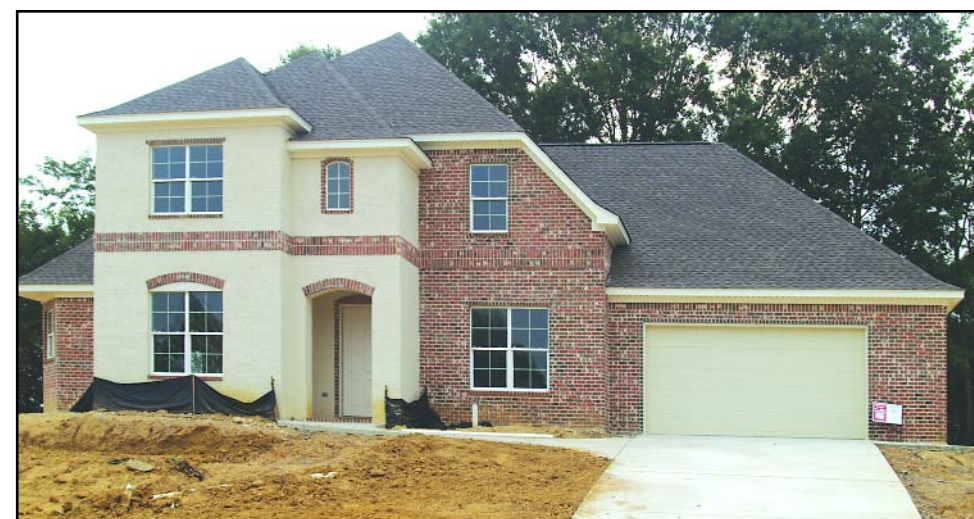
An Energy Star home nears completion in Noblewood Homes' new Glen Arbor residential development, located in the Brandon area on Louis Wilson Road.
