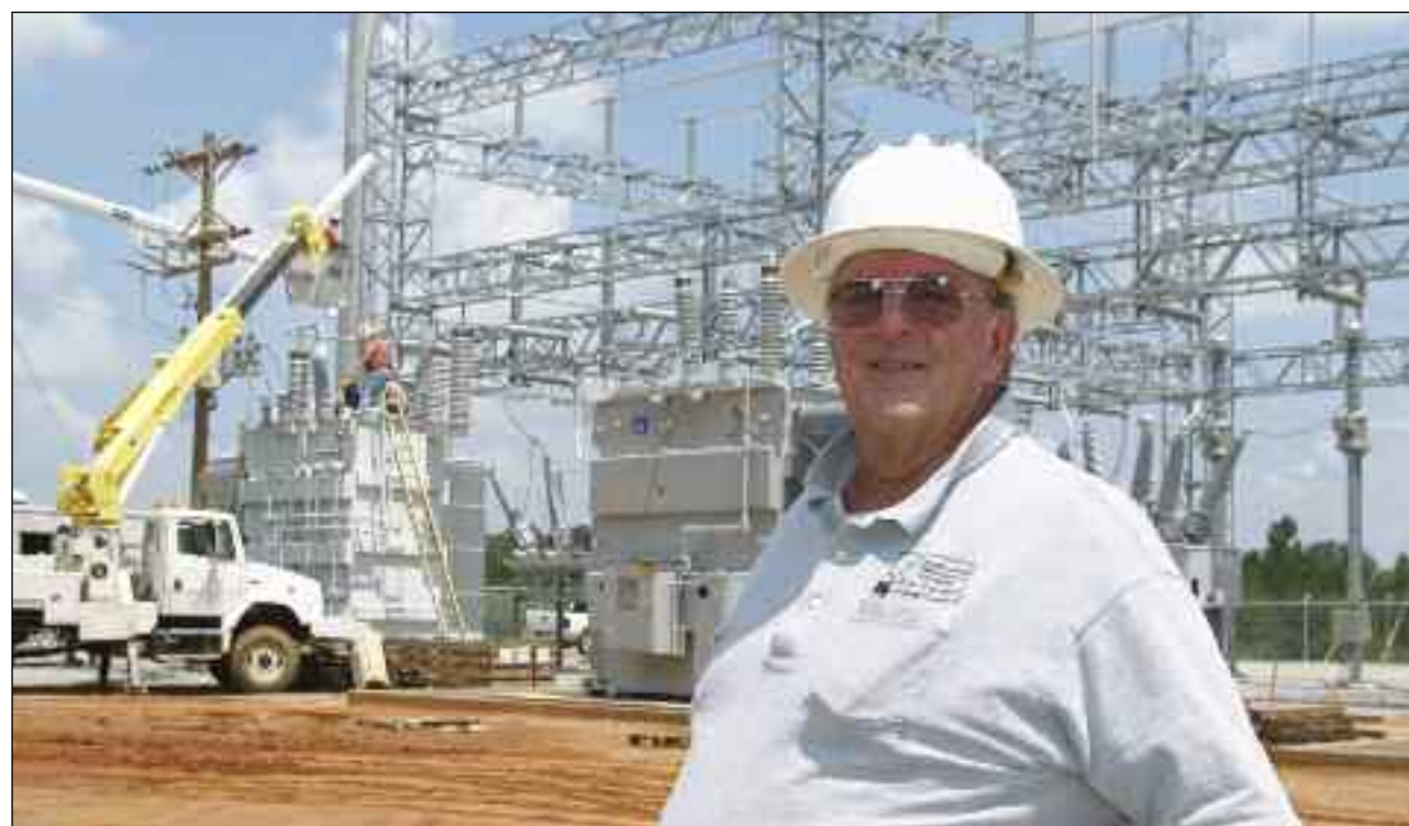
Johnny Barr, Southern Pine construction supervisor, checks on his crew's progress at a new substation nearing completion in Jeff Davis County. The substation will serve the electrical needs of an underground salt-dome natural gas storage facility being developed by Mississippi Hub LLC.
